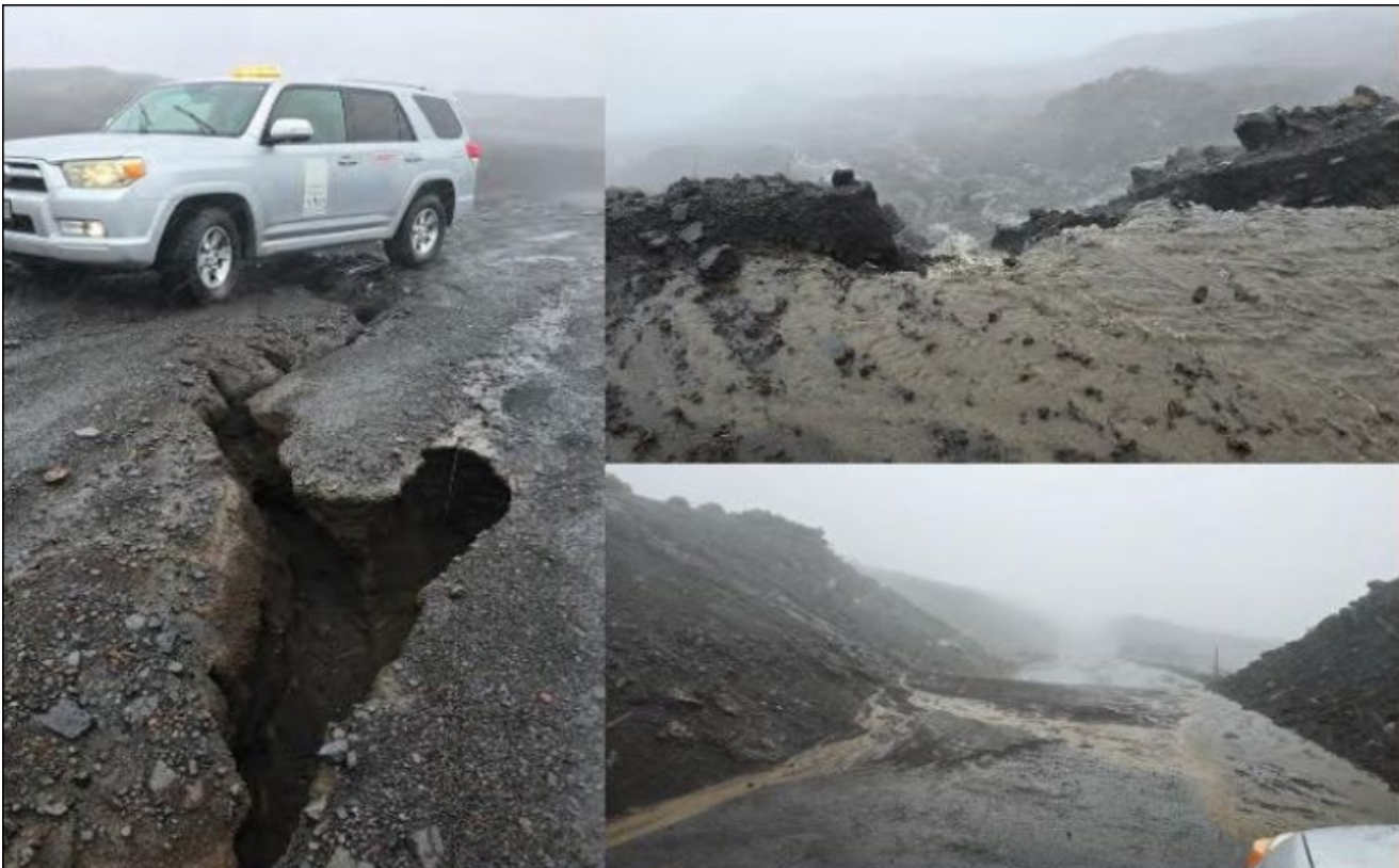
Figure 9. Hurricane Hone Damage.
