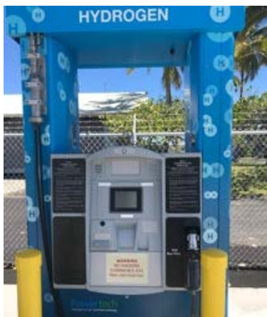
Figure 6. Hydrogen station dispenser.
