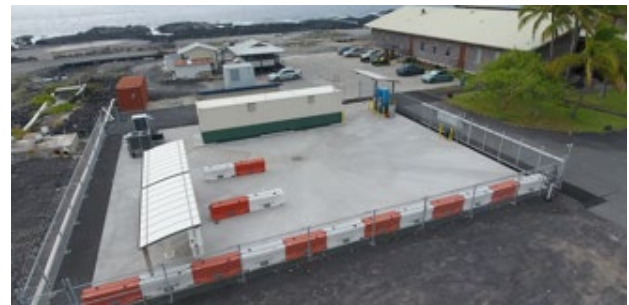
Figure 3. HNEI Hydrogen Station
