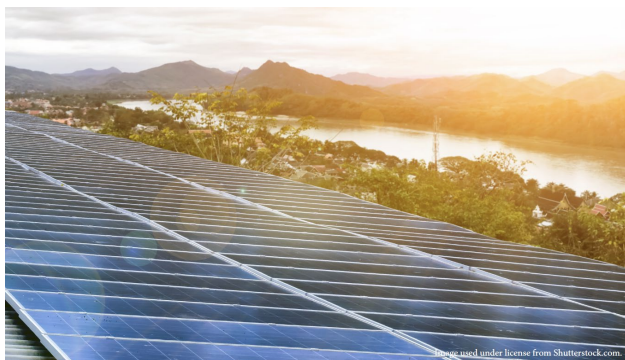
Figure 1. Rooftop solar PV array in Luang Prabang, Laos.
