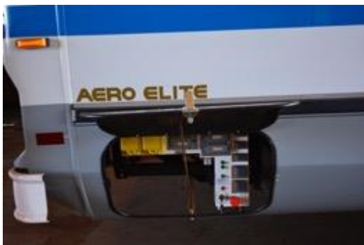
Figure 10: Bus Export Power Unit.
