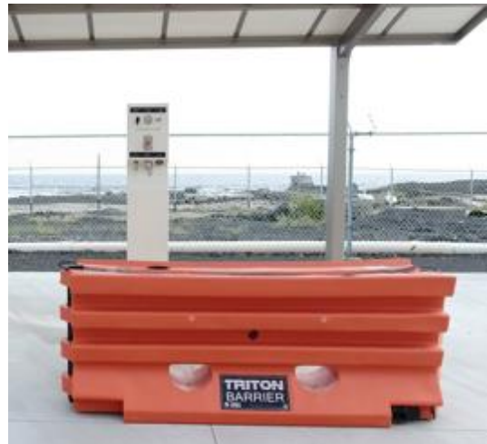
Figure 7: NELHA Fueling Post Interface.
